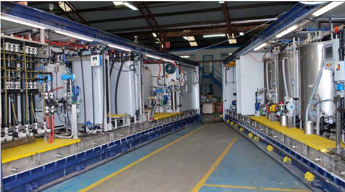
Figure 1 – PhosEnergy Process Demonstration Plant
